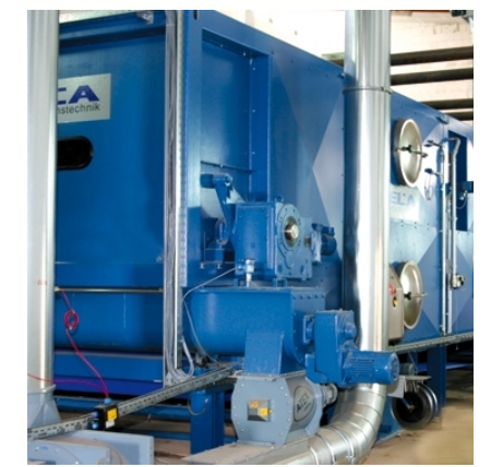
SBT 60 discharge area
